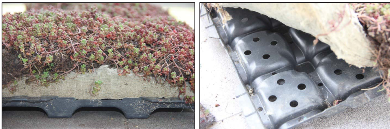
Slika 8: Sestava strehe 2 (vegetacija, substrat, kamena volna, drenaža) (Vir: avtor) Figure 8: Configuration of the roof 2 (vegetation, substrate, rockwool, drainage) (Source: author)
