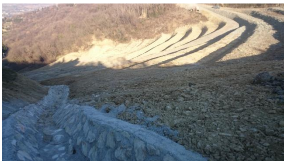
Slika 25: Osrednji del deponije v gradnji (zajeto februar 2015) Figure 25: The central part of the landfill under construction (taken on february 2015)
