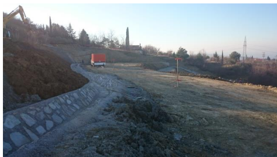
Slika 26: Zgornji del deponije v gradnji na delu predvidene slemenske ceste Jagodje - Šared (zajeto februar 2015) Figure 26: The constuction of the landfill upper part in the area of planned ridge road Jagodje - Šared (taken on february 2015)
