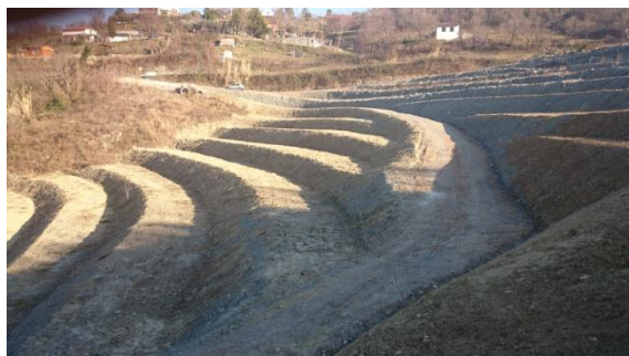
Slika 24: Osrednji del deponije v gradnji (zajeto februar 2015) Figure 24: The central part of the landfill under construction (taken on february 2015)
