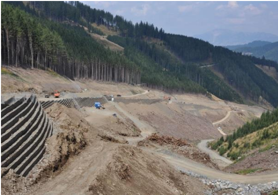
Slika 33: Armirana brežina v gradnji na orografski levi strani deponijskega prostora Figure 33: Prestressed slope under construction on the orographic left side of the landfill area (vir: http://www.hinteregger.co.at/ , 2014)
