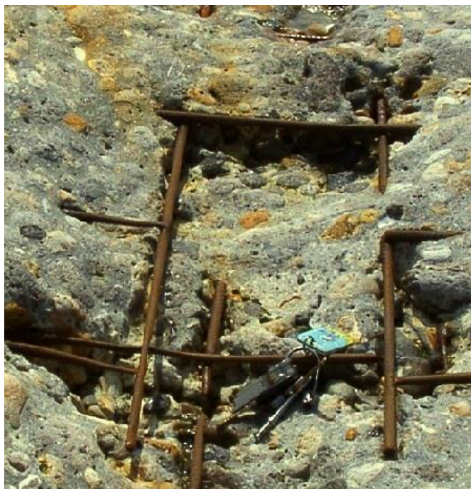
Slika 12: Pojav abrazijske erozije na betonski podlagi (Foundation, Concrete and Earthquake Engineering)
