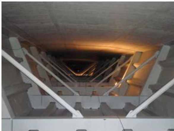
Figure 8: The inside of the structure of the motorway viaduct (Lešnica) with a steel and concrete construction where the system of measuring points was installed for collecting of strain values
