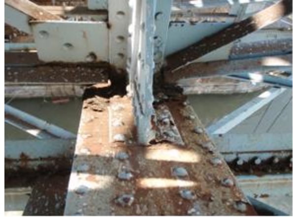
Figure 7: Railway Bridge in Maribor: progressive corrosion on a joint of the vertical, horizontal and diagonal joint elements
