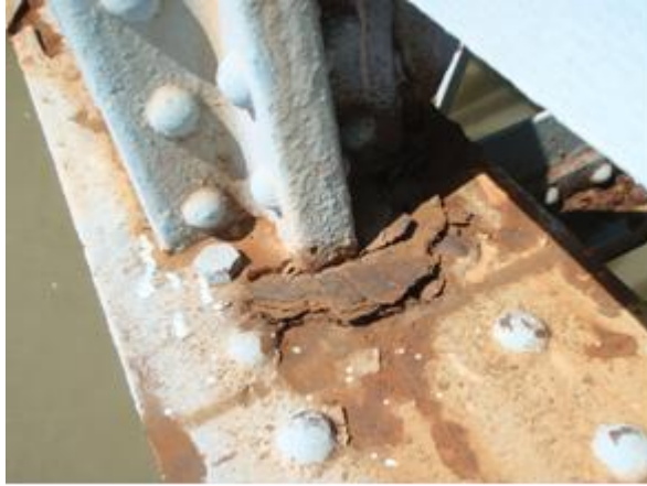
Figure 6: Railway Bridge in Maribor: progressive corrosion on a joint of the main arch girder and vertical element
