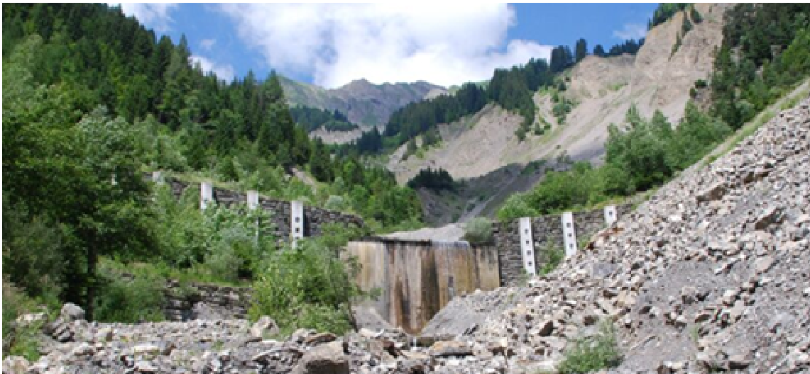
Fig. 5 Check dam IVa with rehabilitation measures, middle part fixed by a concrete plate and pre-stressed anchors in 1976, buttresses and pre-stressed anchors installed at the barrier wings in 2000
