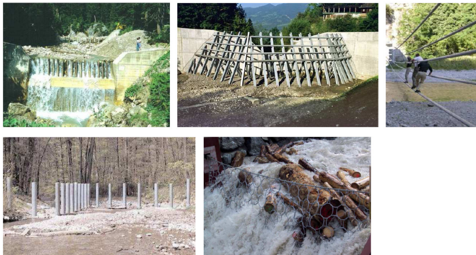
Fig. 1 Images of different types of wood retention structures in the European Alps (higher centered and lower left images are from Lange and Bezzola, 2006; the lower right from Geobrugg, 2007).
