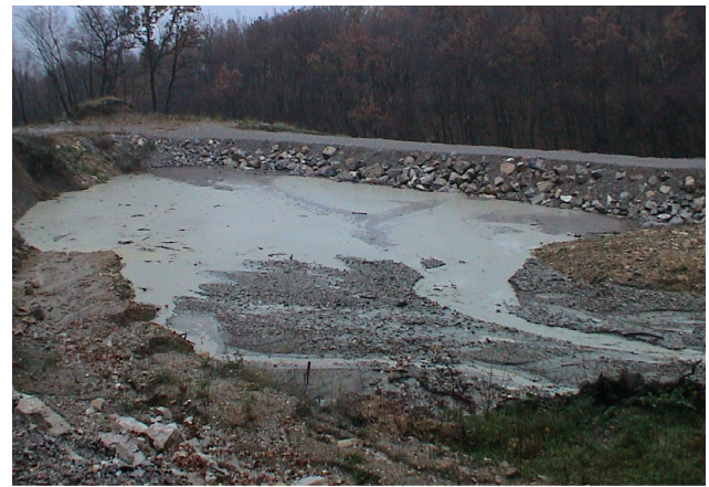
Fig. 8. The rockfill dam that can retain up to 5000 m 3 of mud and debris was constructed to protect the village of Lokavec from extremely rapid mud flows generated at the surface of the stopped earth flow masses.
