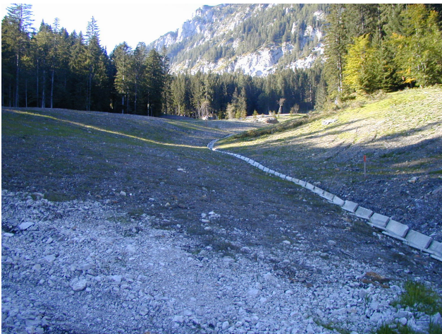
Fig. 15. Stabilised part of the Macesnik landslide above the pontoon bridge by introducing several deep drainages and peripheral and central surface drainage.
