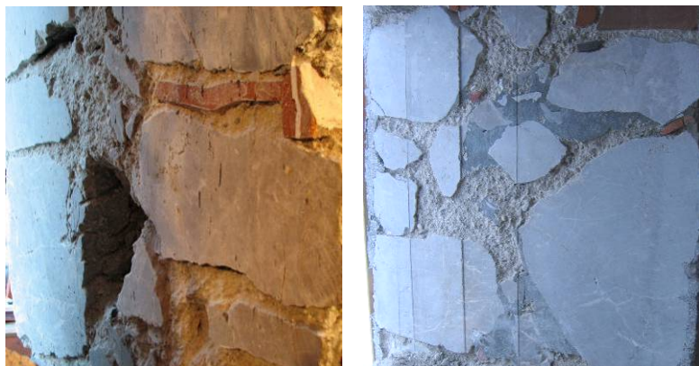
Slika 5.19: Prečni prerez neinjektiranega zidu 6 (levo) in injektiranega zidu 1-C1 (desno) Fig. 5.19: Cross section of the ungrouted wall specimen 6 (left) and grouted wall specimen 1-C1 (right)
