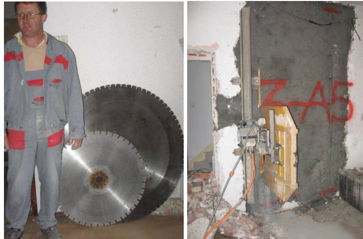
Slika 5.22: Rezanje zidu 3-AC2 z diamantno krožno žago Fig. 5.22: Cutting of the wall 3-AC2 using diamond circular saw
