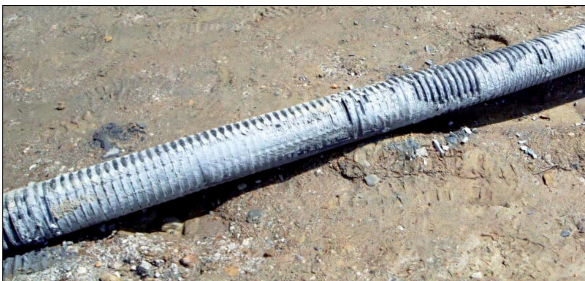
Slika 3.27: Izvlečeno slabo zainjektirano trajno prednapeto geotehnično sidro, vgrajeno pod kotom 5°. Figure 3.27: Pulled-out permanent prestressed ground anchor poorly grouted under angle of 5°.
