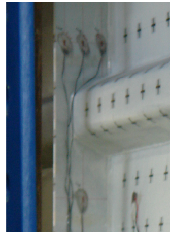
b) Uni-axial strain gauges in the transverse stiffener
