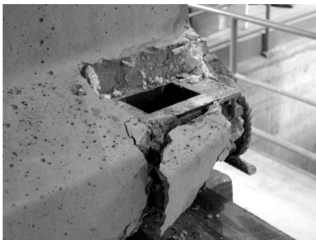
Slika 2.10: Poškodba nosilca na stiku z stebrom Figure 2.10: Damaged beam at the beam-column connection
