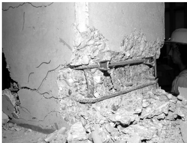
Slika 2.18: Tipična upogibna porušitev stebra Figure 2.18: Typical flexural failure of a column
