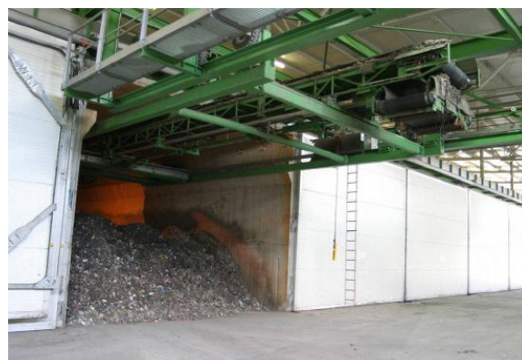
Slika 6: Tunelski kompostirnik Figure 6: The tunnel composter
