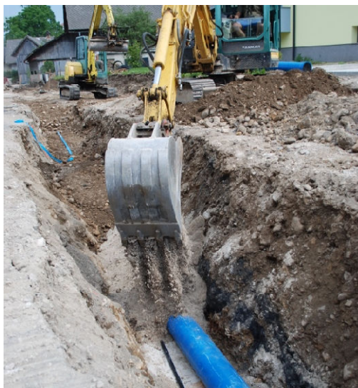
Slika 21 Obsip cevododa s kamenim agregatom 0/4 (kontrolirani pogoji) (Vir: lastni arhiv) Figure 21 Pipe overlay with crushed sand 0/4 mm (Source: personal archive)
