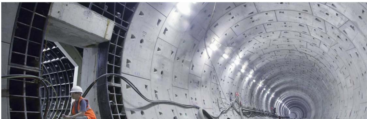
Slika 4-8: Obloga predora iz predizdelanih segmentov s prečnikom (www.crossrail.co.uk). Figure 4-8: Completed segmental lining with cross passage connection (www.crossrail.co.uk).
