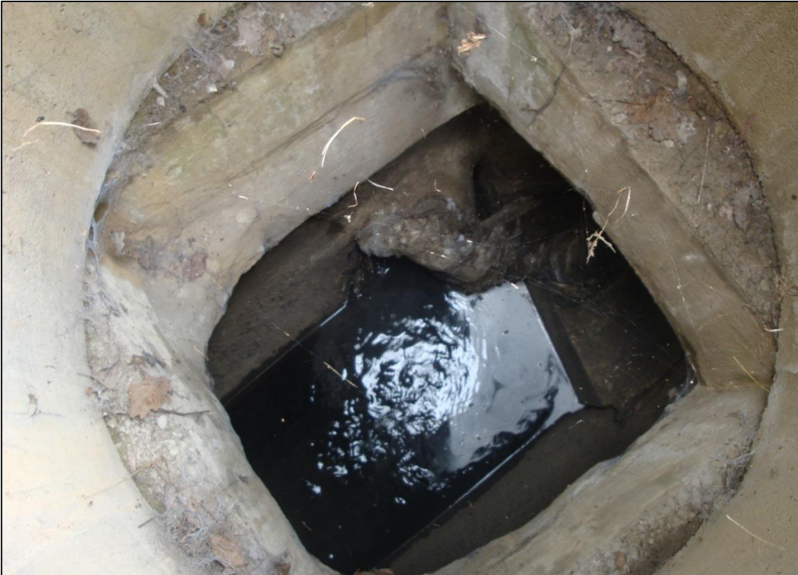
Slika 13: Razbremenilnik s prelivnim robom brez potopne stene – RA 5 (osebni arhiv). Figure 13: Stormwater overflow without weir – RA 5 (personal archive).
