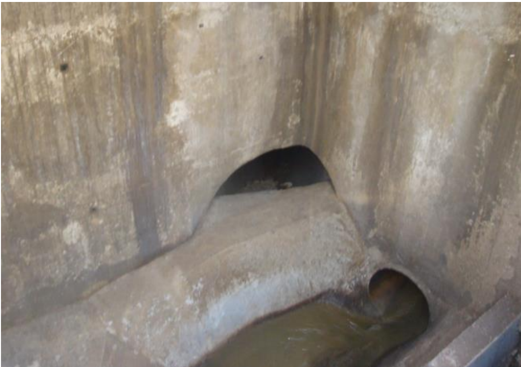
Slika 17: Razbremenilnik pred ZB 5 – pogled na blindiran vtok v zadrževalnik (osebni arhiv). Figure 17: Stormwater overflow before ZB 5 – view at the closed inflow into the stormwater tank (personal archive).
