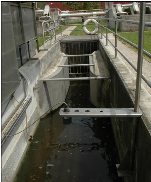
Slika 24: Primer vgradnje Khafagi – Venturijevega preлива na CČN Domžale (osebni arhiv). Figure 24: Example of installation Khafagi – Venturi flume on WWTP Domžale (personal archive).
