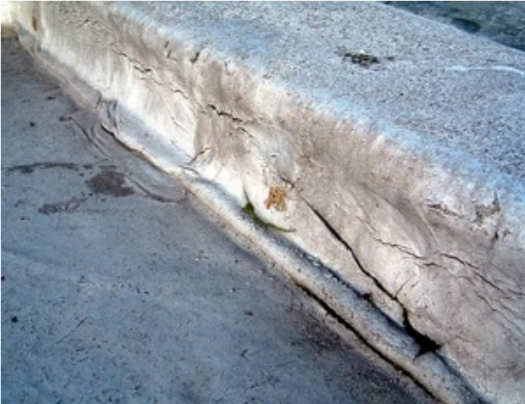
Slika 29: Zgrbančenje asfalta in razpoke (when flat roofs fail, 2016).
