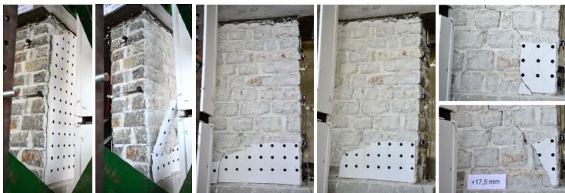
Figure 3.75: Detachment of the plaster prior its collapse and its subsequent collapse at test 8 - SNv-15-1 Slika 3.75: Odstopanje ometa pred porušitvijo in postopna porušitev pri testu 8 - SNv-15-1
