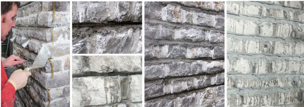
Figure 4.17: Cords placed into the joints with cement-lime mortar, cord placed into the groove with cement-lime mortar (upper) and with epoxy mortar over epoxy primer (bottom), with cement-lime mortar repointed joints and with epoxy mortar repointed joints (from left to right)
