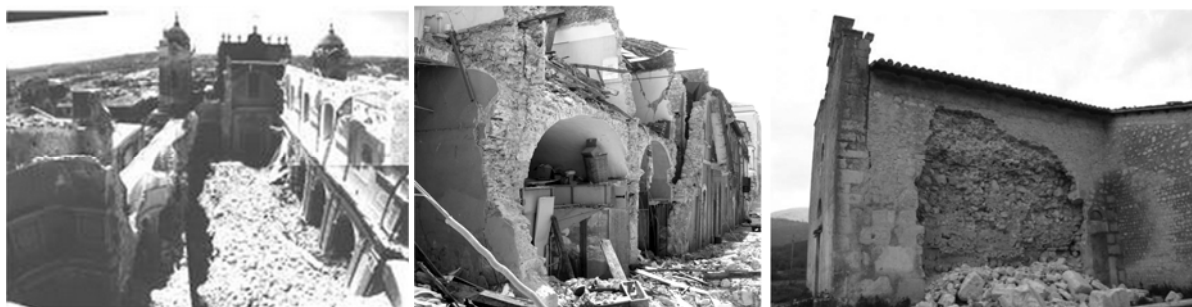
Figure 1.2: Ruins of the Noto Cathedral after 1996 collapse [5] (left), out-of-plane failure mechanism due to poor connection of the structural elements (middle, http://db.nzsee.org.nz/Seminars/2014/Lagomarsino_Wellington_2014-2-20.pdf ) and out-of-plane collapse of masonry wall due to poor connection of the masonry [6] (right) in L'Aquila, Abruzzo, Italy
