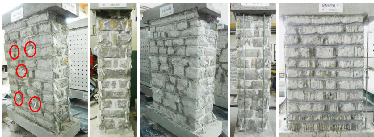
Figure 4.19: Retrofitted and NSM strengthened walls Slika 4.19: Injektirani in z vrvicami v fugah utrjeni zidovi
