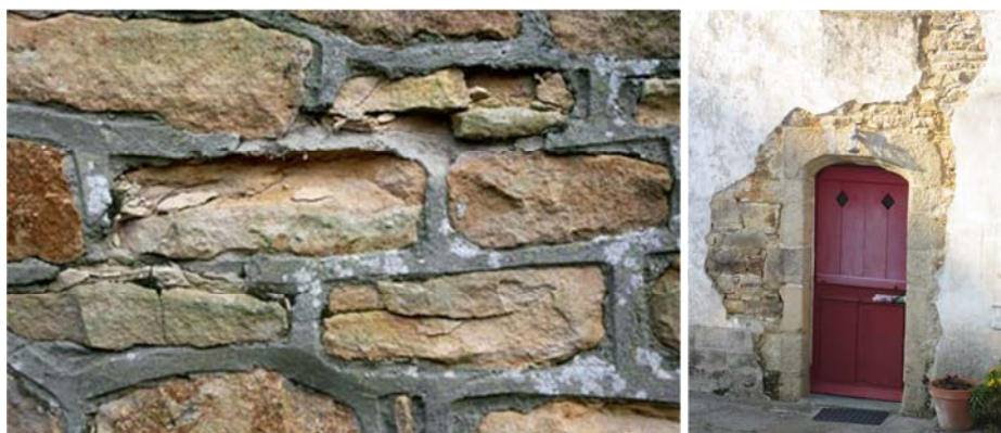
Figure 1.5: Spalling as a result of cement mortars used for pointing (left, http://www.periodliving.co.uk/renovation/expert-advice/interior-wall-maintenance ), delaminating cement render over granite and clay mortared walls on a part of the 16 th century manor in St Jean du Doight, Bretagne, France (right, https://jontybarrett.wordpress.com/vernacular/traditional-building-methods/ )
