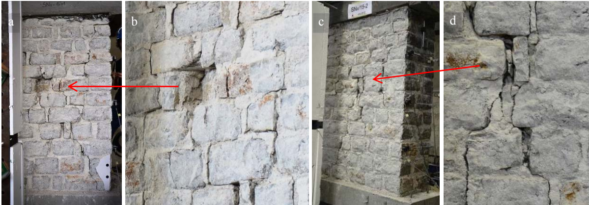
Figure 3.35: Crack pattern on the walls after test 8 - SNv-15-1 (a, b) and test 10 - SNv-15-2 (c, d) Slika 3.35: Poškodovanost zidov po testu 8 - SNv-15-1 (a, b) in testu 10 - SNv-15-2 (c, d)
