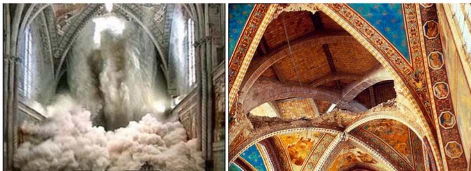
Figure 1.4: Collapse of the St Francis of Assisi Basilica ceiling during 1997 Umbria-Marche earthquakes (left, http://projecthistoryitalia.altervista.org/26-settembre-1997-terremoto-nelle-marche-e-in-umbria/ ), destroyed Cimabue fresco vault ceiling in the Assisi Basilica (right, http://it.wikipedia.org/wiki/File:Volta_Cimabue.jpg )
