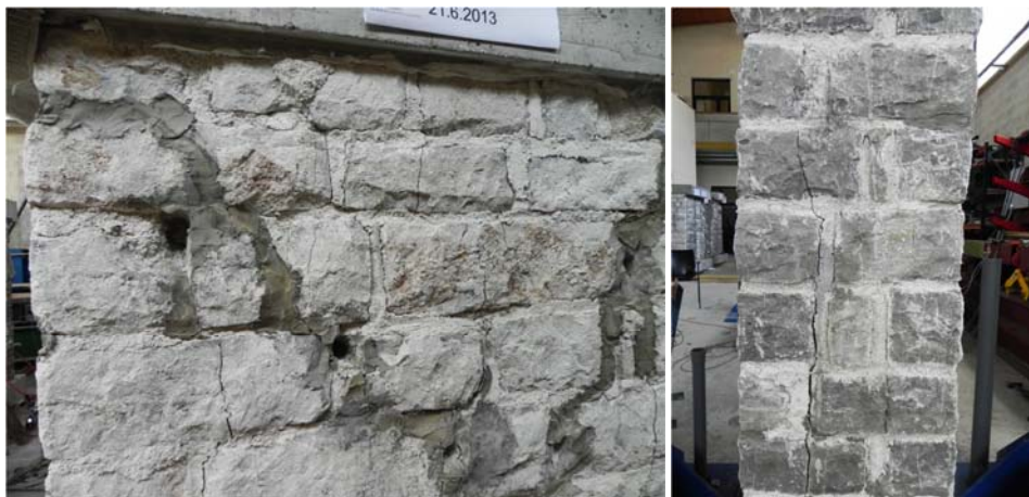
Figure 5.2: Damage pattern after failure attained at test T1 - I(n) Slika 5.2: Poškodovanost zidu po testu T1 - I(n)
