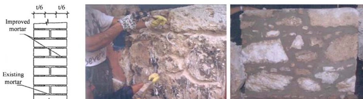
Figure 2.25: Deep repointing of brick (left, adapted from [168]) and of stone masonry (middle and right) [170] Slika 2.25: Prefugiranje opečne (levo, prilagojena [168]) in kamnite zidovine (na sredini in desno) [170]
