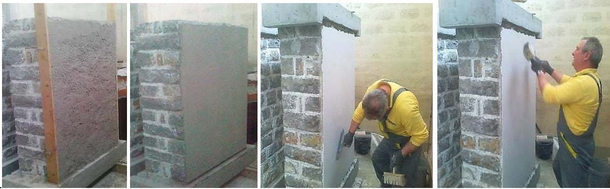
Figure 3.4: Application of the coarse (left two photos) and fine (right two photos) plaster [43]
