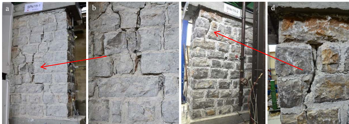
Figure 3.36: Crack pattern on the walls after test 12 - SPk-15-1 (a, b) and test 14 - SNk-15-2 (c, d) Slika 3.36: Poškodovanost zidov po testu 12 - SPk-15-1 (a, b) in testu 14 - SNk-15-2 (c, d)
