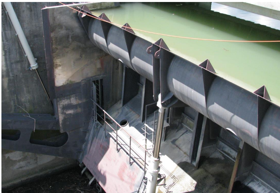
Slika 11: HE Vrhovo – segmentna zapornica z zaklopko Figure 11: HPP Vrhovo – radial/tainter gate with flap
