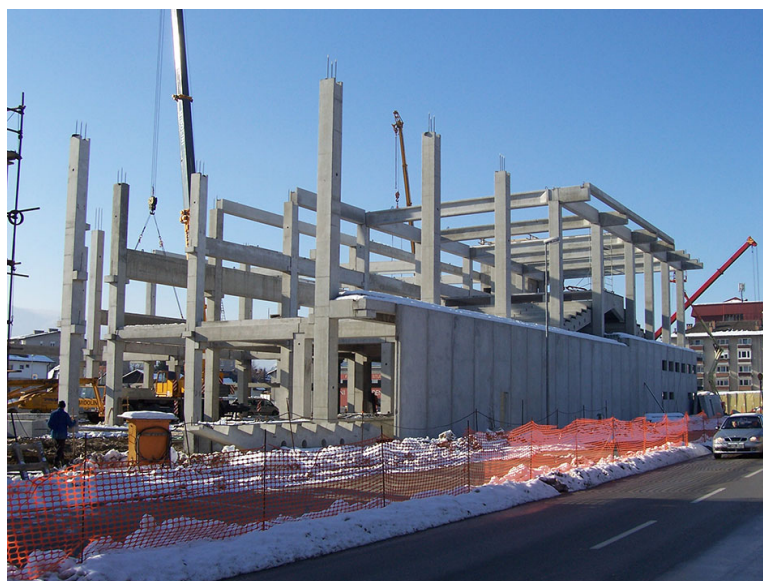
Fig. 1 The most commonly used structural system for precast industrial buildings in Europe consists of an assemblage of slender cantilever columns, which are tied together by beams
