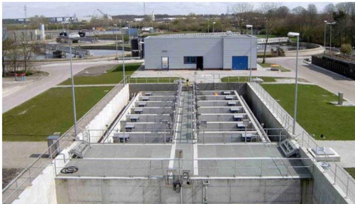
Slika 48: Filtri s tkanino na CČN Oldenburg ( Q_{max}= 5.800 \text{ m}^3/\text{h} ) Figure 48: Cloth filters on WWTP Oldenburg ( Q_{max}= 5.800 \text{ m}^3/\text{h} )
