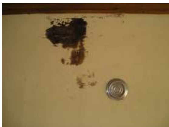
Slika 9: Vlaga zaradi zamakanja dimnika (Bartol-Pohl in sod., 2006)
