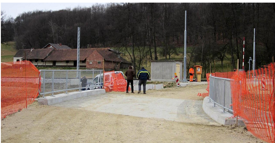
Slika 46: Območje naleganja prekladne konstrukcije pred in po izvedbi integriranega zveznega prehoda Figure 46: Bridge superstructure ,positioned on abutment, before and after construction of the integrated approach
