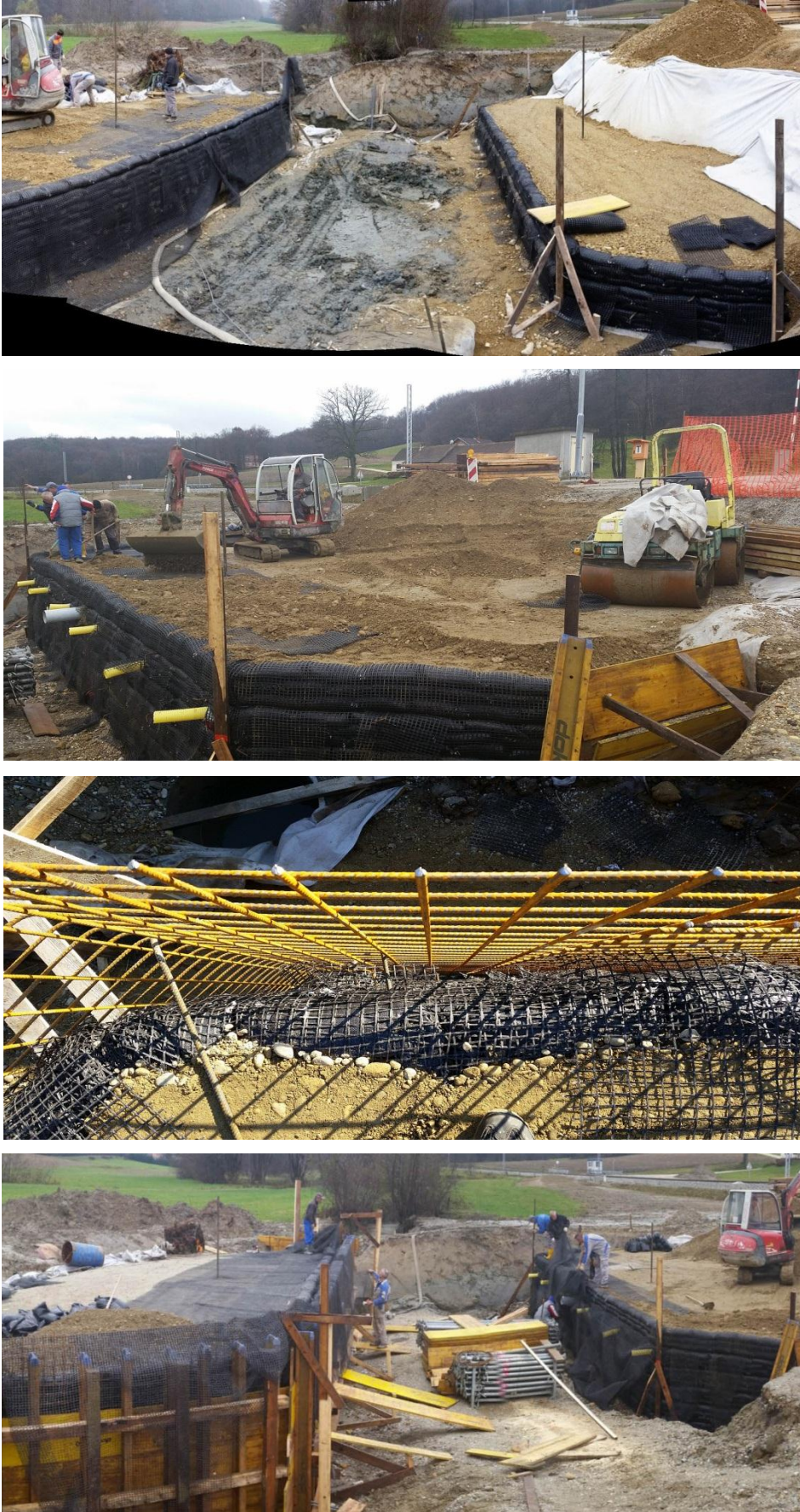
Slika 44: Posamezne faze gradnje opornika iz armirane zemljine Figure 44: Some construction phases of the GRS abutment
