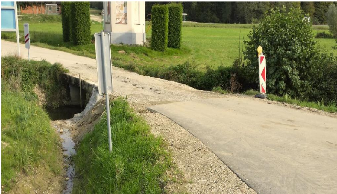
Slika 15: Most v Žerovincih pred rekonstrukcijo Figure 15: Existing bridge in Žerovinci before reconstruction
