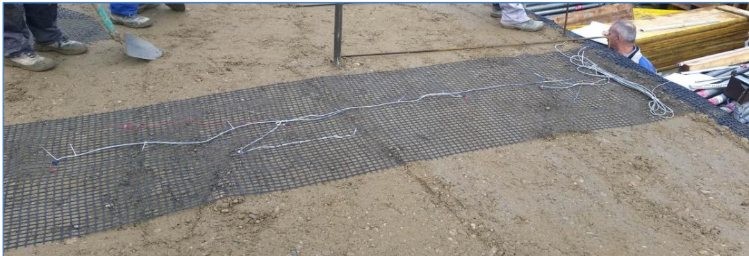
Slika 51: Vgrajena geomreža z merilnimi lističi Figure 51: Built-in geogrid, equipped with strain gauges
