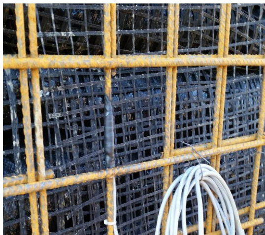
Slika 52: Vgrajena armaturna mreža z merilnimi lističi Figure 52: Facing structure reinforcement, equipped with strain gauges
