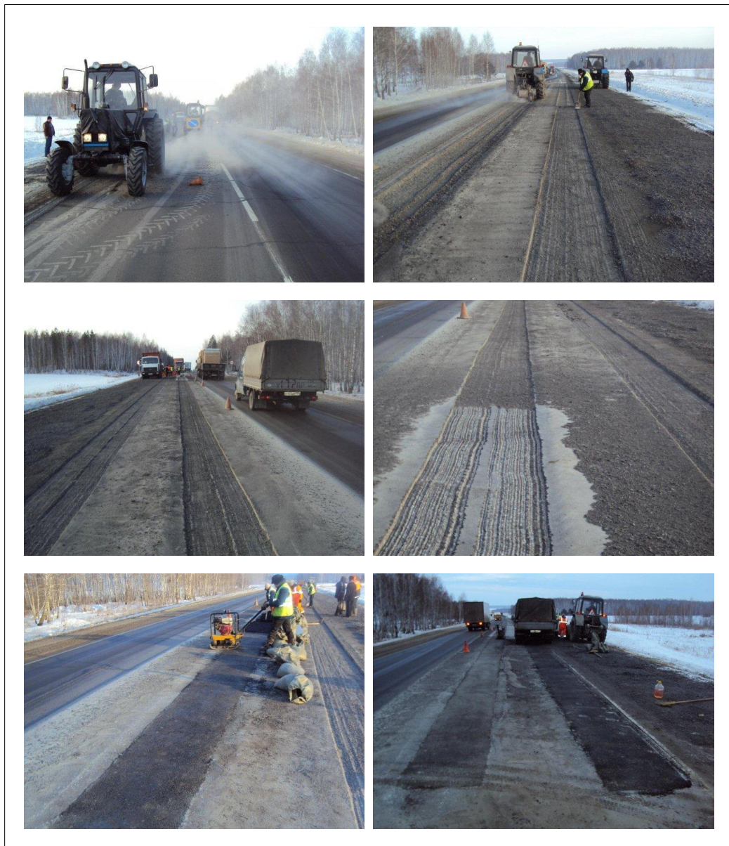
Slika 44: Sanacija kolesnic na cesti Federal Highway M5, December 2010 – Chelyabinsk, Russia (Cantat Associates Inc., 2012) [22]
