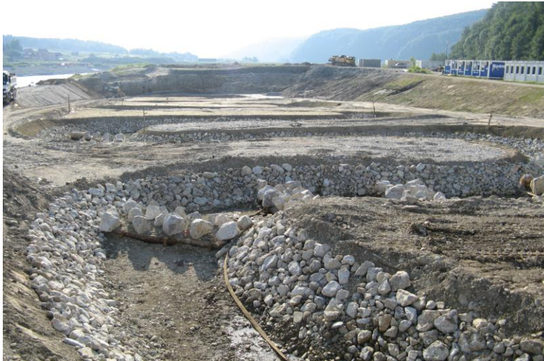
Slika 13: HE Blanca – obhodni kanal (z uravnavanjem dinamike vodnega toka). Figure 13: HPP Blanca – bypass fishway (with levelling water flow dynamics).
