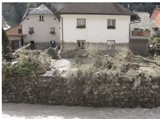
Fig. 5. Flood trace on a building used for peak water level assessment in Železniki (photo: Urban Ilc).
