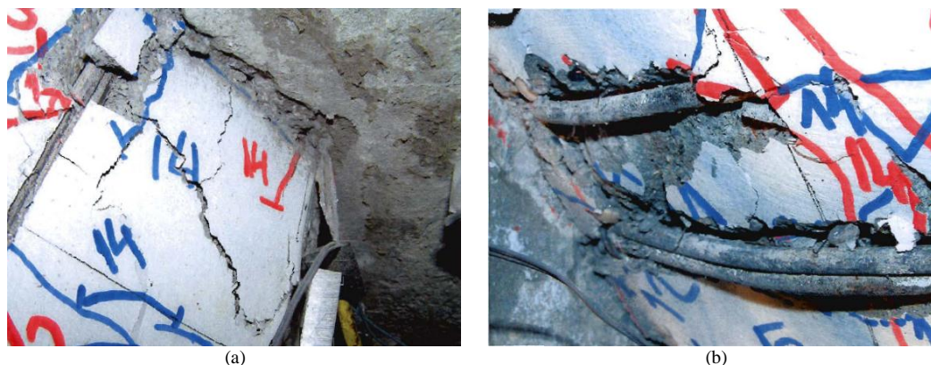
Slika 3.19: (a) Drobljenje betona in (b) uklon armaturnih palic ob vpetju stebra v petnajsti fazi Figure 3.19: (a) Concrete crushing and (b) reinforcement buckling at pier base in fifteenth phase
