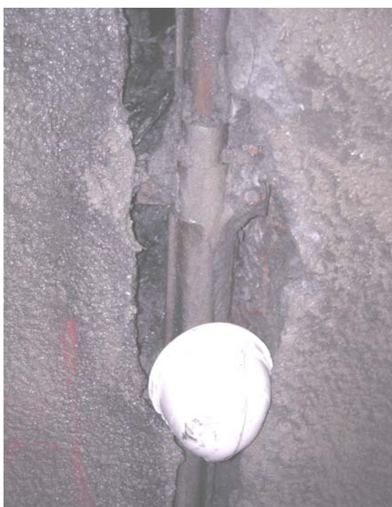
Figure 5-25. Photo of large crack in primary lining of the right tube of the exploration gallery due to excessive longitudinal displacements.
