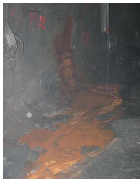
Figure 5-16. Ferric hydroxide in tunnel waters.
